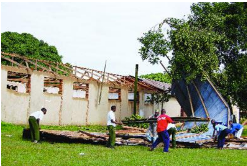
Above is a photograph showing school building whose roof came off due to heavy rainfall
